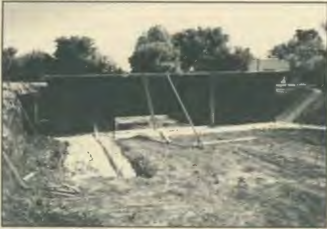
Our new home is being built within sight of our main monastery. Constructed below ground level, this space will ultimately become our garage/storm shelter.
