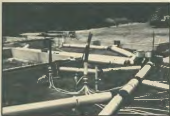
Air conditioning/heating duct work rests in the red clay subflooring of the house.
