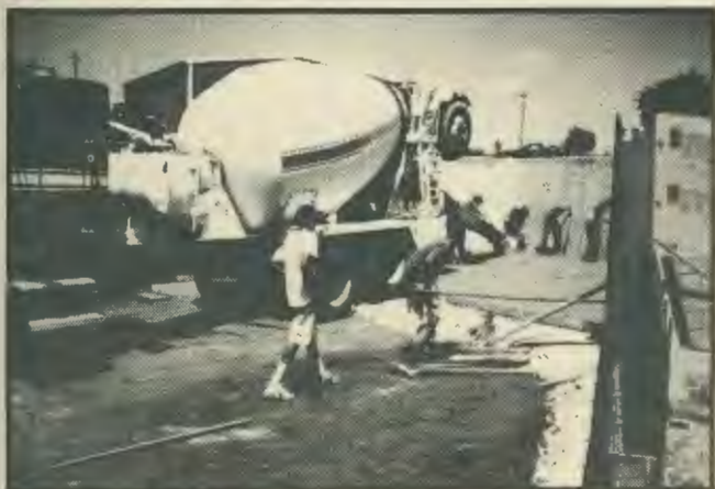
Hard working crews pour the cement flooring on a sweltering summer day -- temperature 105 degrees°.
